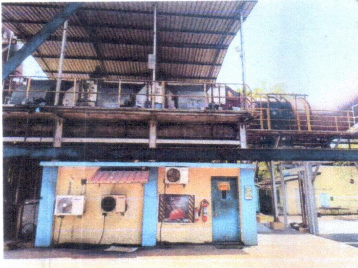
Image : Onsite Photograph of Bag Filter Unit installed for Kiln.
