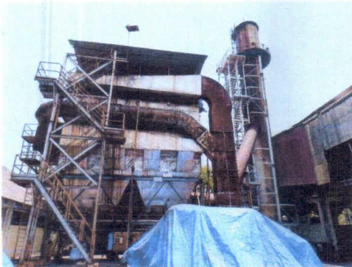
Image : Onsite Photograph of Dust Extraction System (DES).
