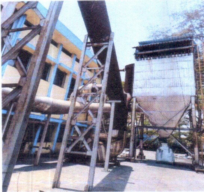
Image : Onsite Photograph of Bag Filter Unit installed for Cooler.
